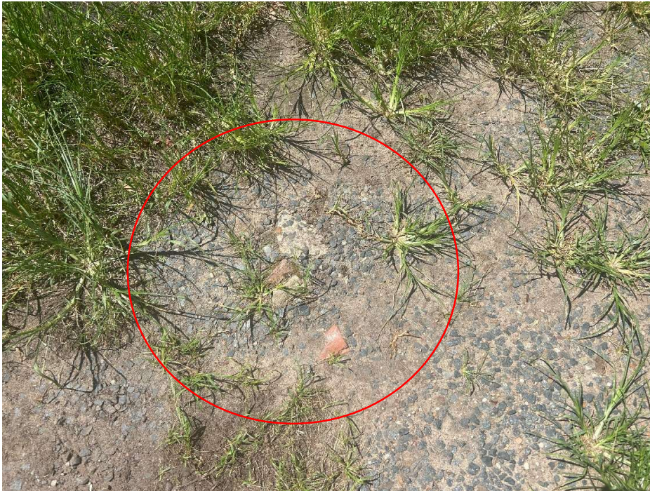
Plate P9. Building rubble observed within the southern portion of 548-550 Box Road
