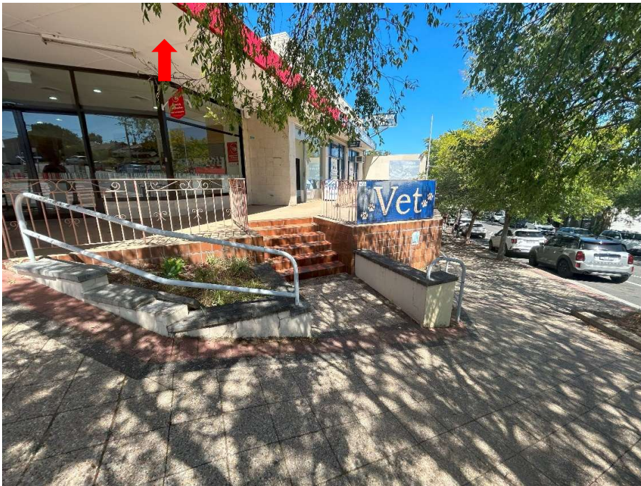
Plate P1. Front of 544-546 Box Road, facing west, potential ACM observed in eaves
