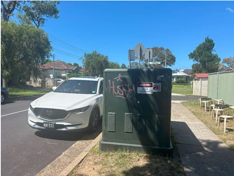
Plate P15. Transformer adjacent to the Site
