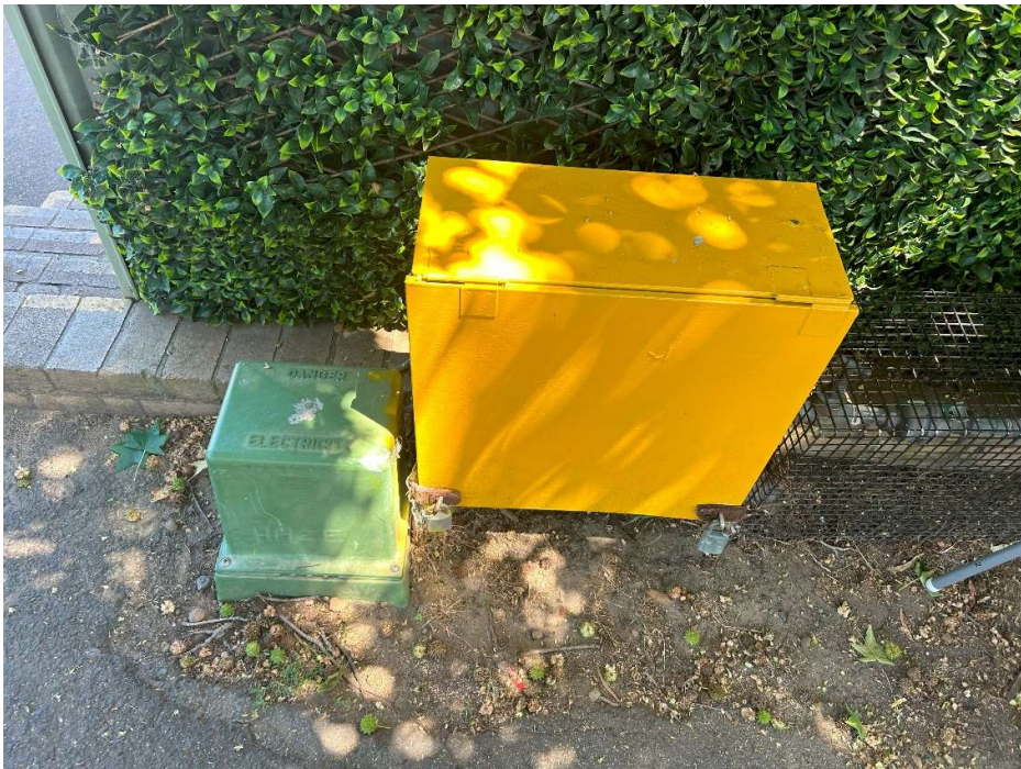
Plate P16. Small electrical box adjacent 544-546 Box Road
