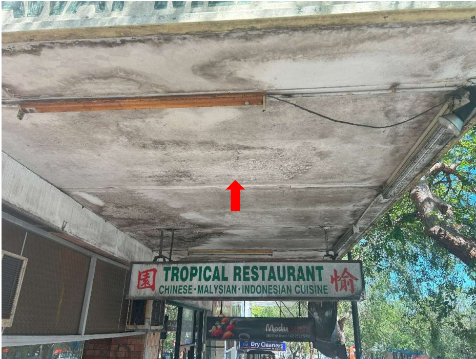
Plate P7. Suspected ACM and peeling paint in eaves of 548-550 Box Road
