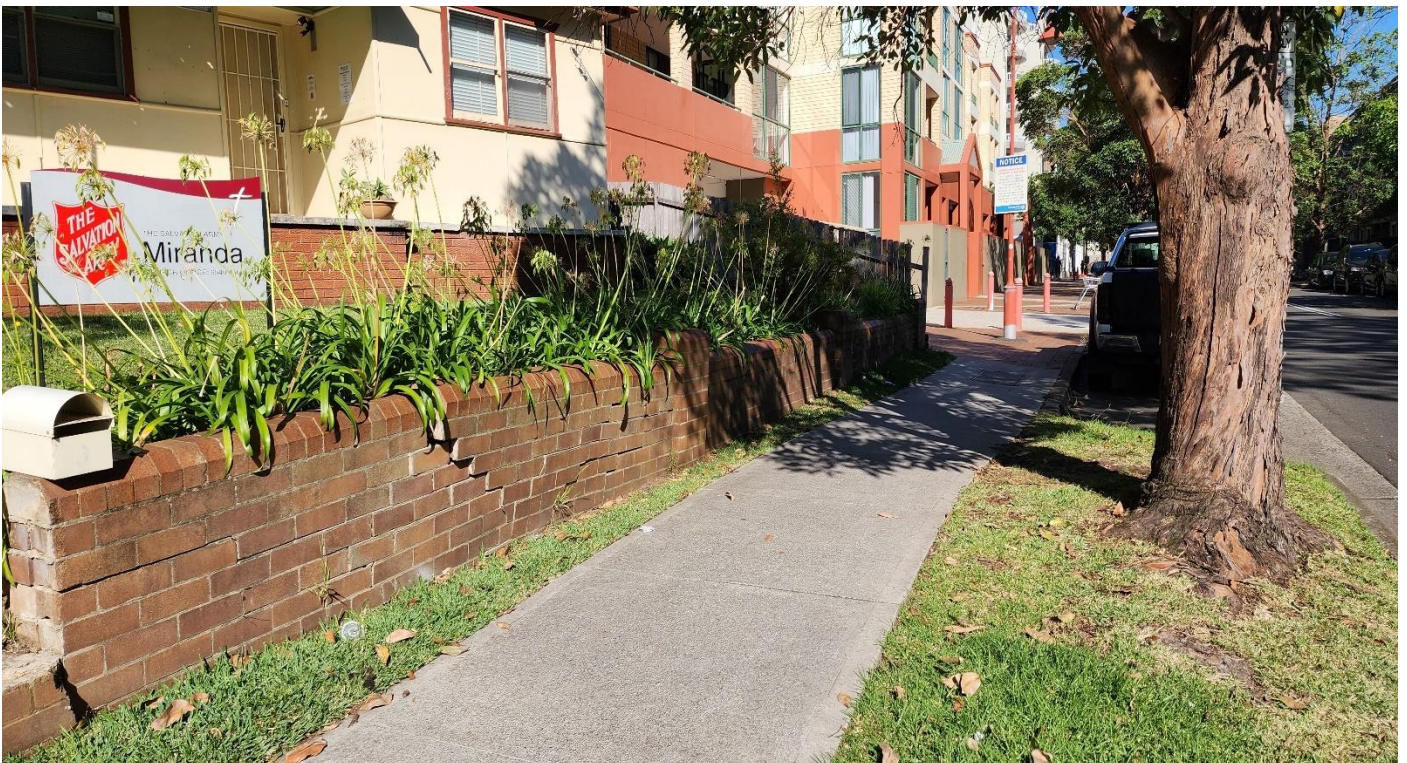
Photograph 10, looking West at boundary wall, fronting tree 11. Structurally dangerous with soil levels within site, much higher than Council verge.
