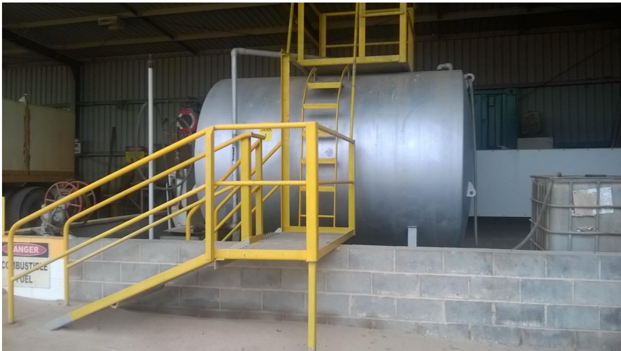
Photograph 10: Diesel AST within bunded area.
