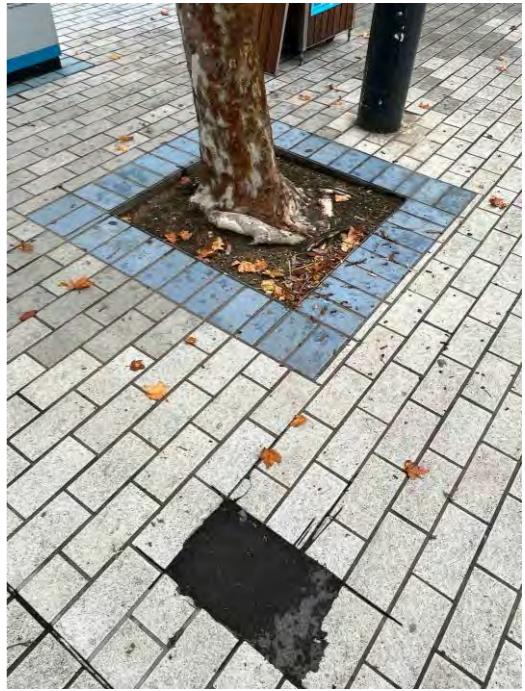
Photograph 17: Soil around trees and patching of brickwork with asphalt in Site 1 area
