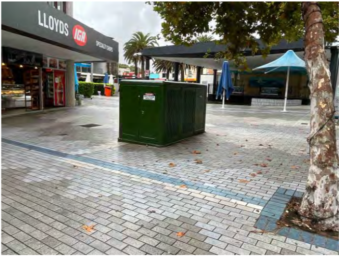
Photograph 16: Pad mount transformer to west of Site 1
