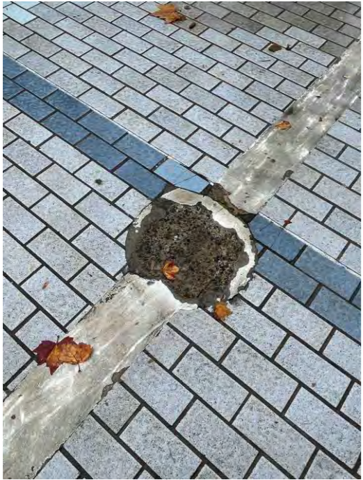
Photograph 18: Repair to brickwork from relocation of shop awning structures in Site 1 area.
