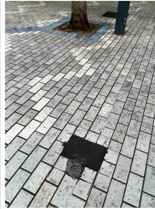
Photograph 24: Soil around trees and asphalt patching on brickwork in footprint of Site 2 area
