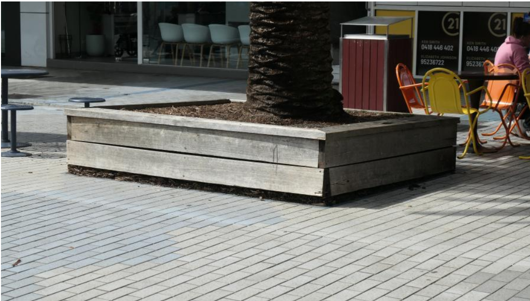
Figure 8 – View of the Phoenix palms at the southern end of the Mall where they have been planted within a raised timber surround. Roots are readily seen around the edges and are lifting the timberwork above the pavement. This is symptomatic of a tree with limited soil volume and indicating that the root mass has most likely fully exhausted the available soil resources and now expanding in the only way it can. (Photo: Arterra 19.9.19)
